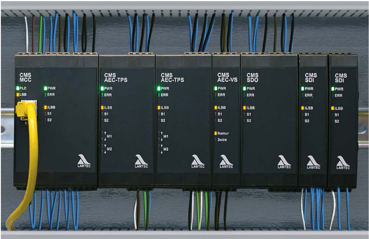
CMS in operation
