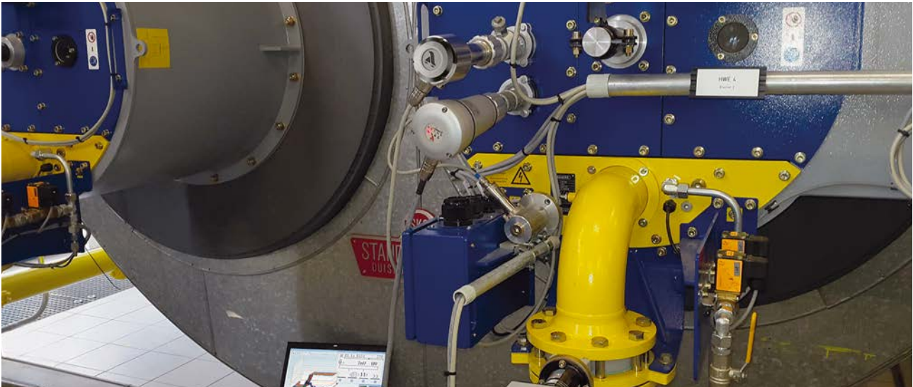
The LAMTEC F300K flame monitoring system in operation
